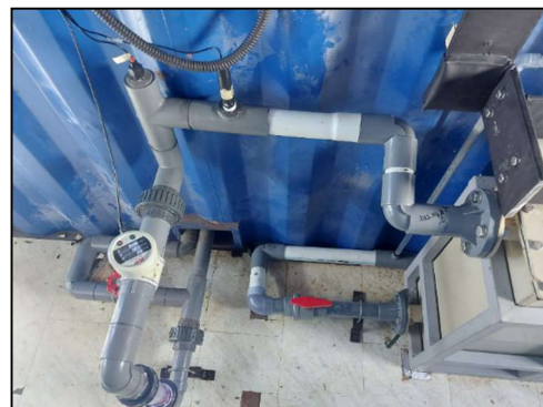
Piping Inlet Reaktor
