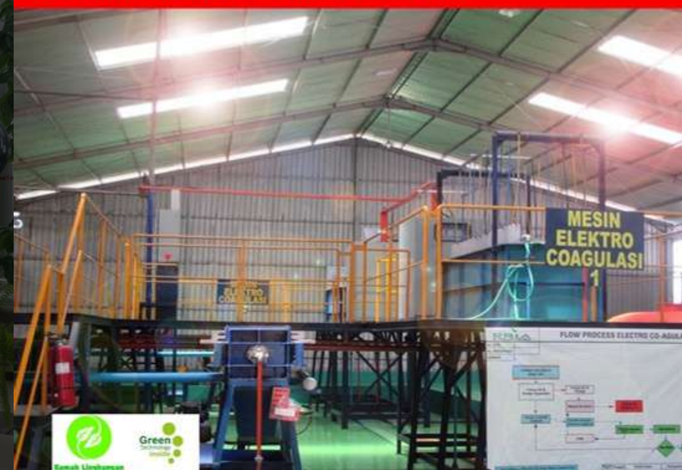
WASTE WATER TREATMENT PLANT - ELECTROCOAGULATION SYSTEM
